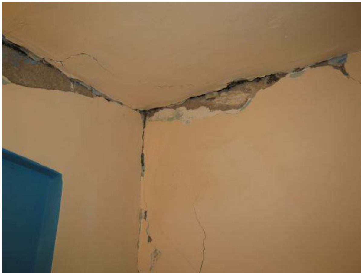
Slika 3. Široke in globoke razpoke na stičiščih nosilnih sten in stropov (foto: Matjaž Godec) Figure 3. Wide and deep cracks on the contacts of load-bearing walls and floors (Photo: Matjaž Godec)
