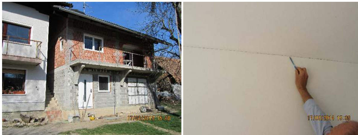
Slika 2. levo: Stanovanjski objekt v vasi Seč; desno: Lasasta razpoka v stiku stene in stropa v tem objektu (foto: Matjaž Godec in Polona Zupančič) Figure 2. left: Building in the village Seč; right: Hair-line crack between wall and ceiling in this building (Photo: Matjaž Godec and Polona Zupančič)
