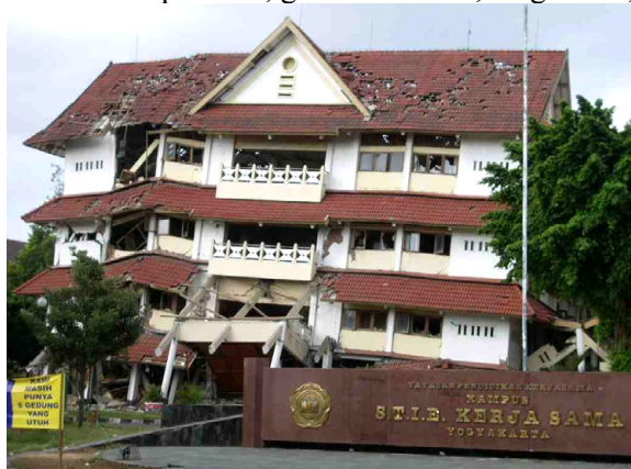
Slika 3. Porušena zgradba šole v Bantulu, južnem delu centralnega dela Jave Figure 3. Collapsed school in Bantul, south part of the central Java
